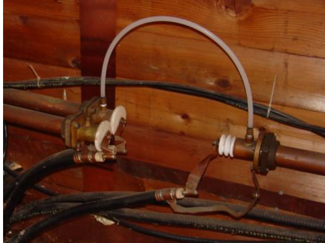
Figure 14.52: Flexible coaxial cables connected to rigid lines.
