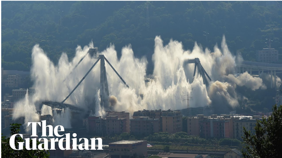
Ponte Morandi [1], Genoa, August 2018 the bridge collapse and 43 persons died. But this is the controlled demolition of June 2019, one year after.
