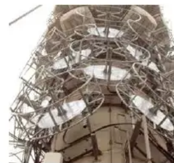
FM circularly polarized antenna system as an array of back-cavity unitary radiators
